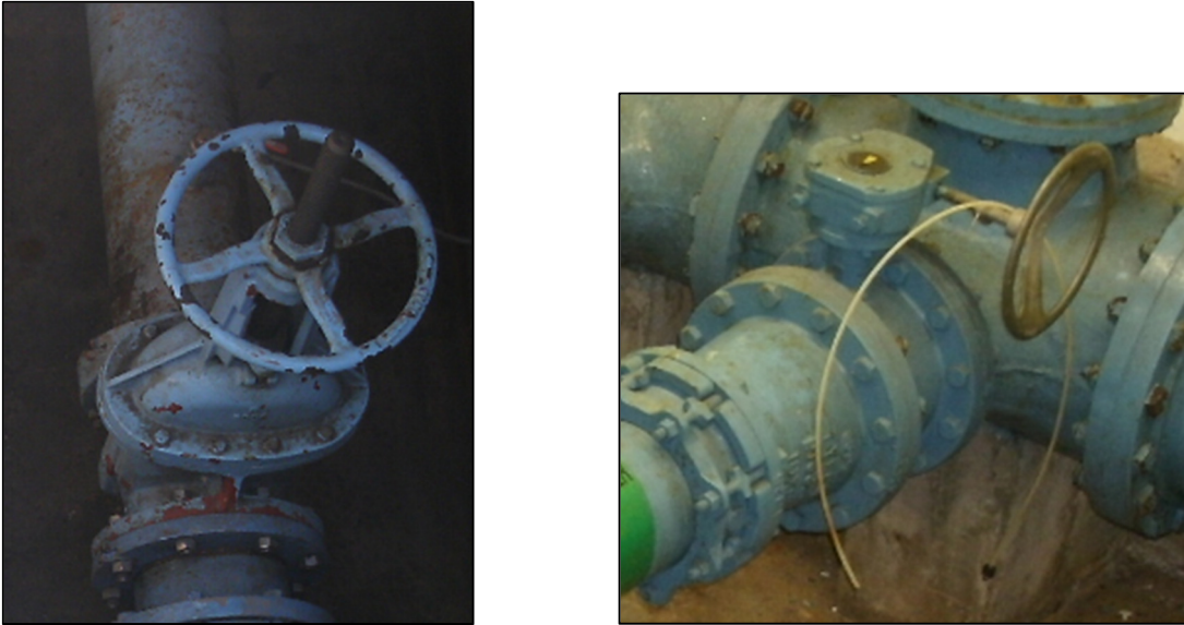
Figure 7-2 Isolation Valves (Two Photographs)
