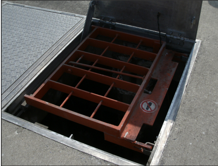
Figure 7-1 Palace Road PS – Safety Grate (Photograph)
